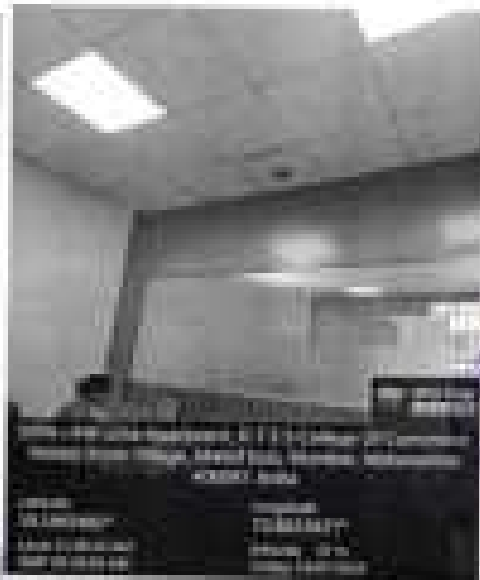
Fire Alarm System
